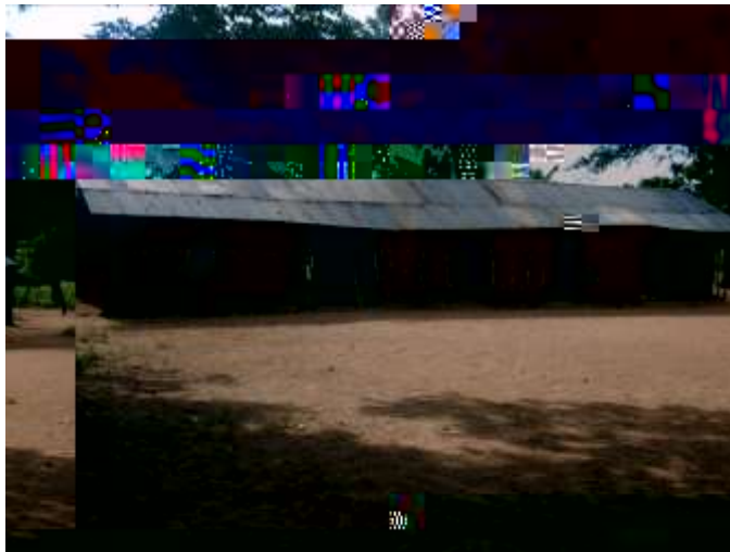
Photo 4: Poor Condition of School Buildings: Nsogolo Primary School, Urambo District.
